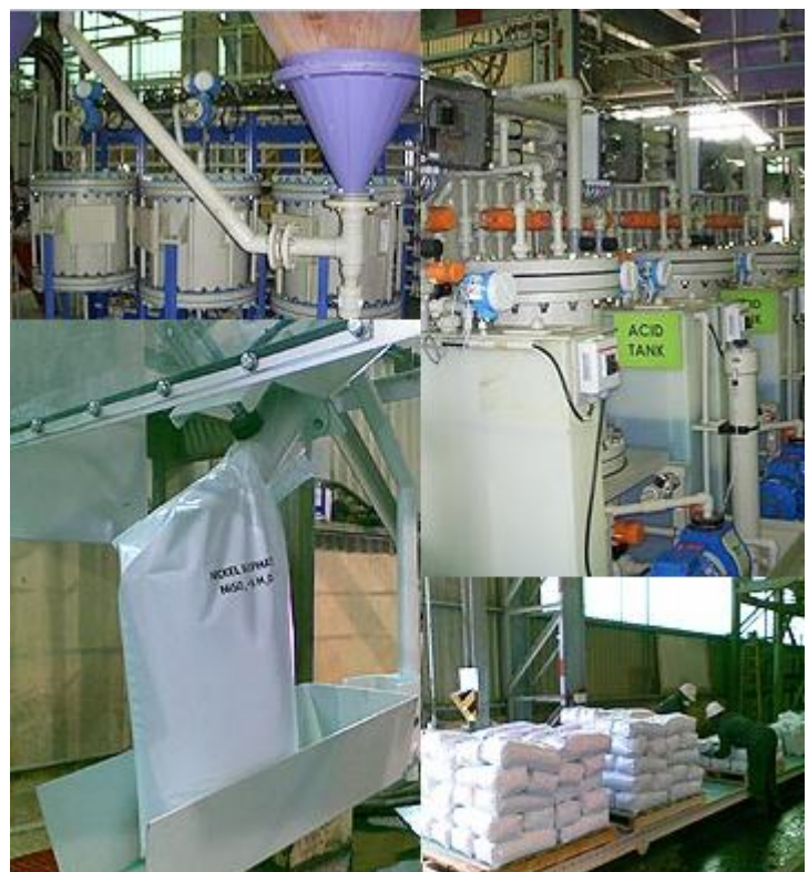
Figure 3: MFC's Palabora nickel extraction plant in Africa is now up and running. Source: wise-owl.com, MFC.
